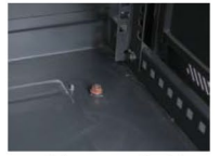
• earthing screw inside
